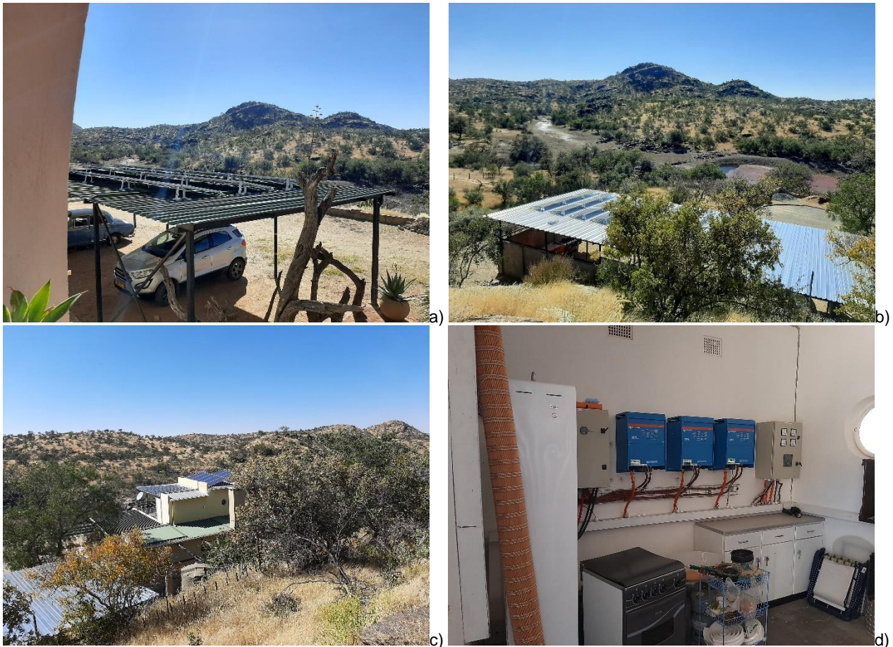
Figure 7: Pictures showing: a) solar panels on the roof of the guest parking area; b) solar panels on the roof of the main house parking area; c) solar panels on the roof of the kitchen/main house area; and d) the control room (Source: L. Maartens, 09 June 2020).
