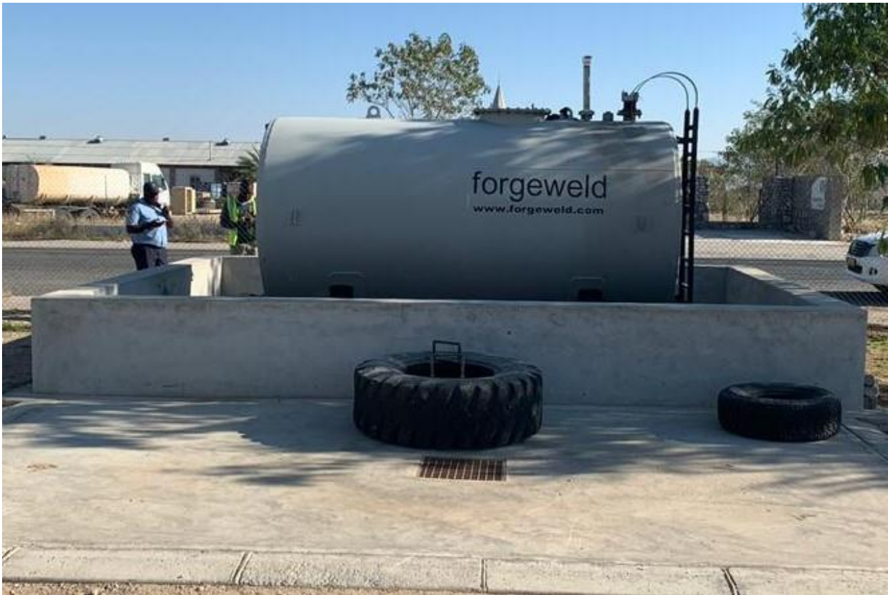
Figure 4. An above fuel tank at Karibib Police Station (photo for illustration purposes only)
