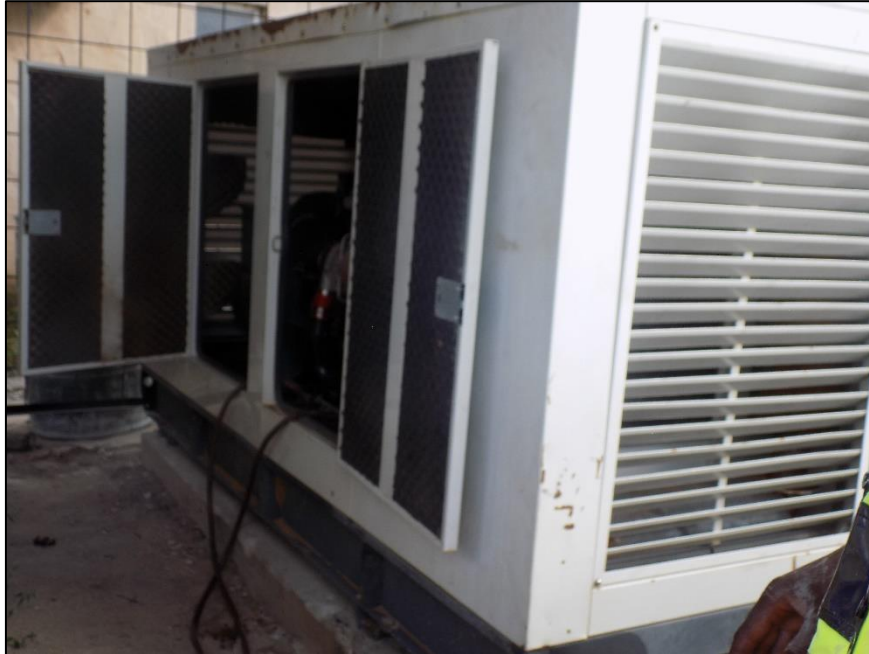
Figure 1-4: Generator at the site
