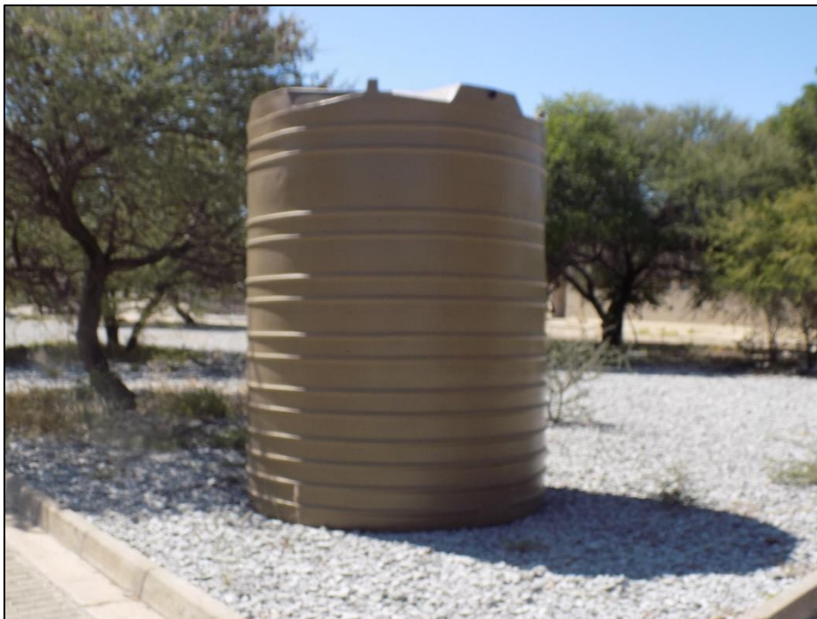
Figure 1-4: Water Storage Tank
