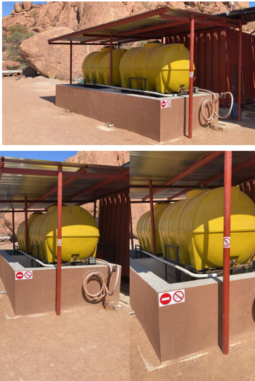
Figure 6-1: The fuel tanks depicting the catchment housing in case of spills, where the capacity is greater than that of the tanks
