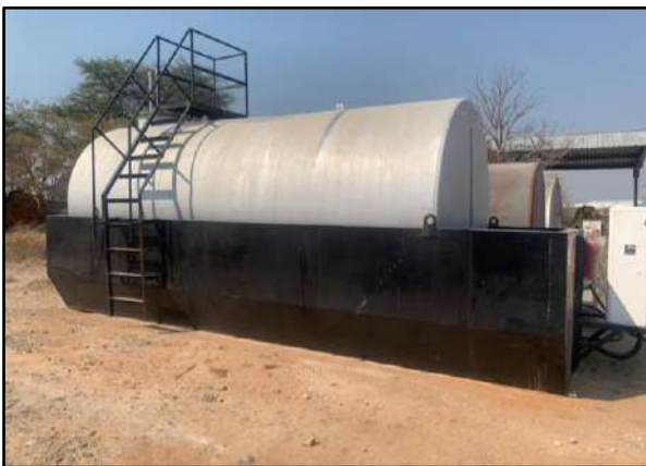
Figure 5: Tank Bund View
