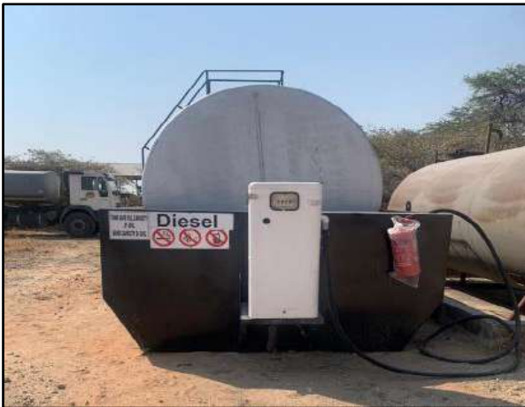
Figure 3: Tank & Related Equipment
