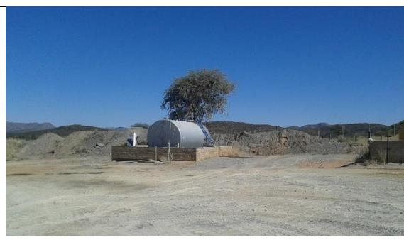
Photo 4. Diesel Refuelling Tanks
