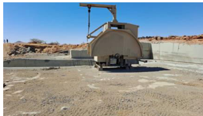
View of blade saw used in developing the eastern test quarry. The test quarry is currently about 2.5m – 3m deep
