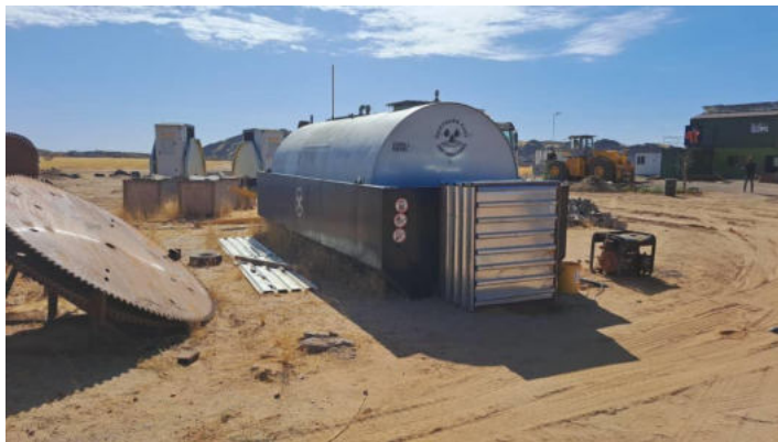
23000L diesel storage tank with dispenser for fuel supply to site machinery. Note that the tank is contained in a steel bund to prevent leakages to ground
