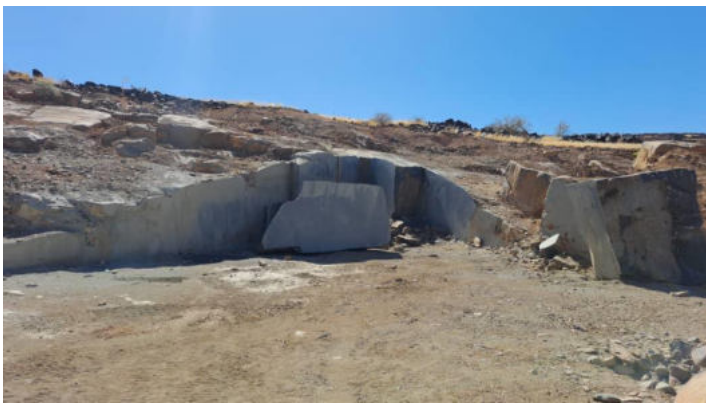
View of 3m deep butterfly cut in dolerite at the western test quarry
