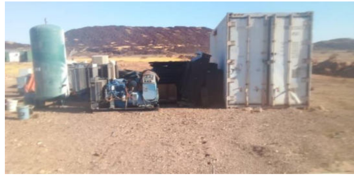
Spares container and equipment spares outside the spare container. Note that there is no concrete lining/ bund
