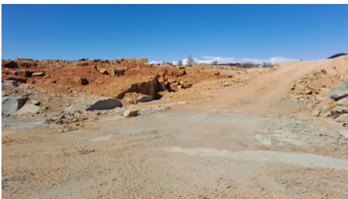
View of north-eastern access ramp into eastern test quarry and area stripped for overburden and loose dolerite boulders
