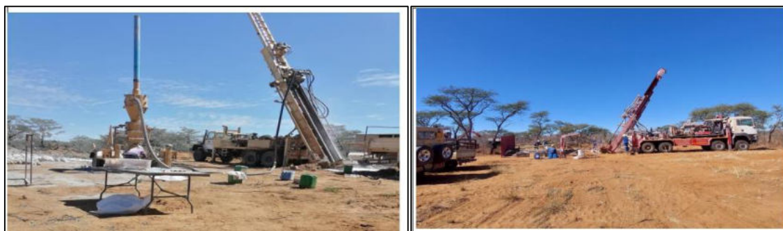
Figure 2-4: A drill rig on an EPL in the Omaheke Region (Resilient Environmental Solutions, 2022)
