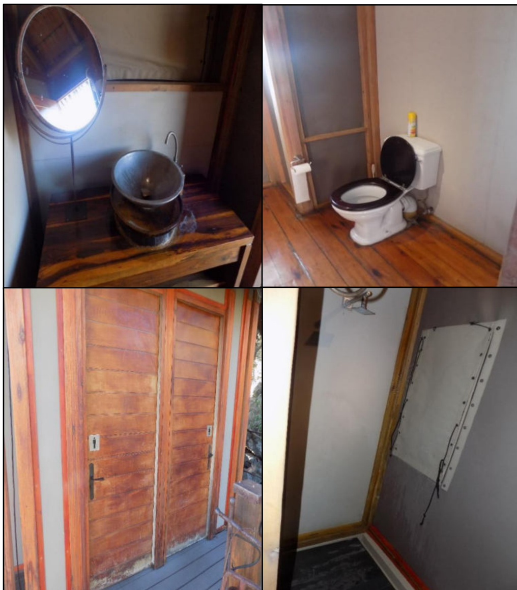
Figure 1-6: Ablution facilities on site
