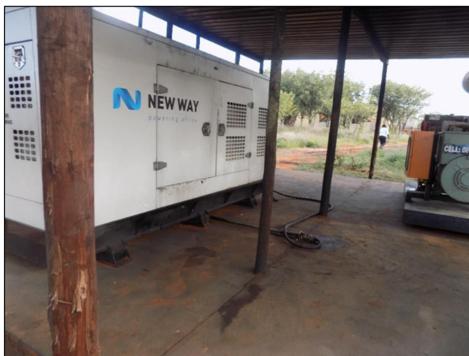
Figure 1-5: Generator on site
