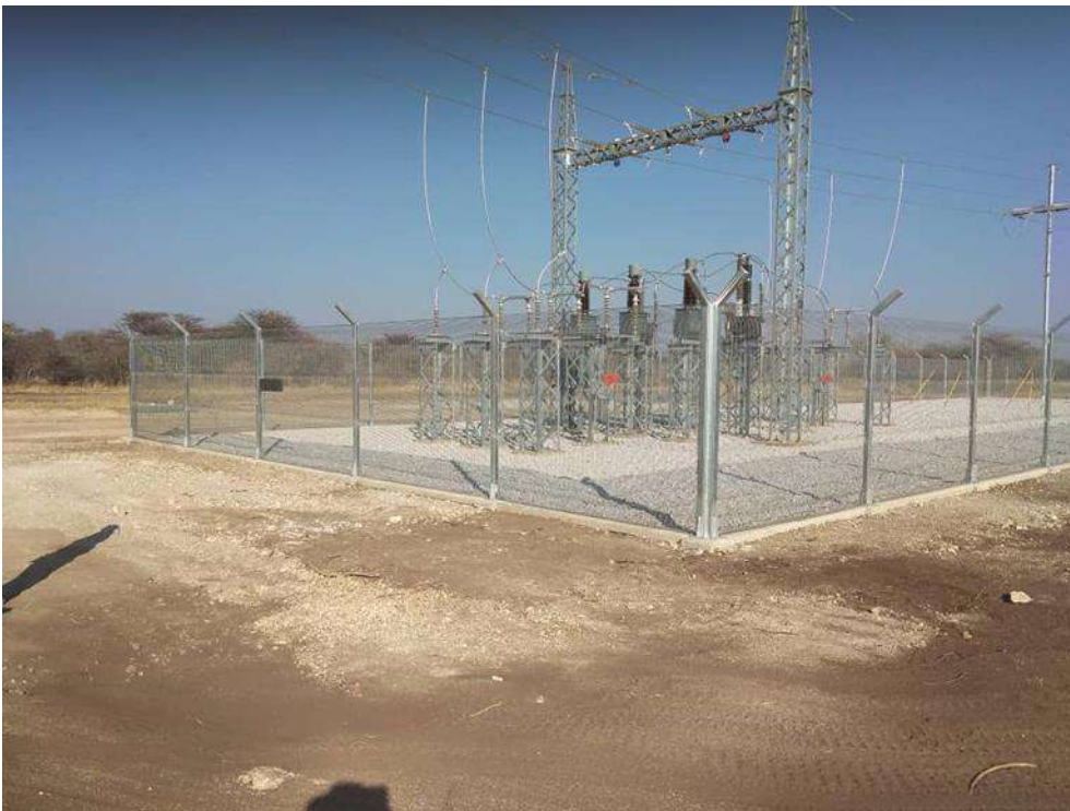
Figure 5 - An example of a metering station
