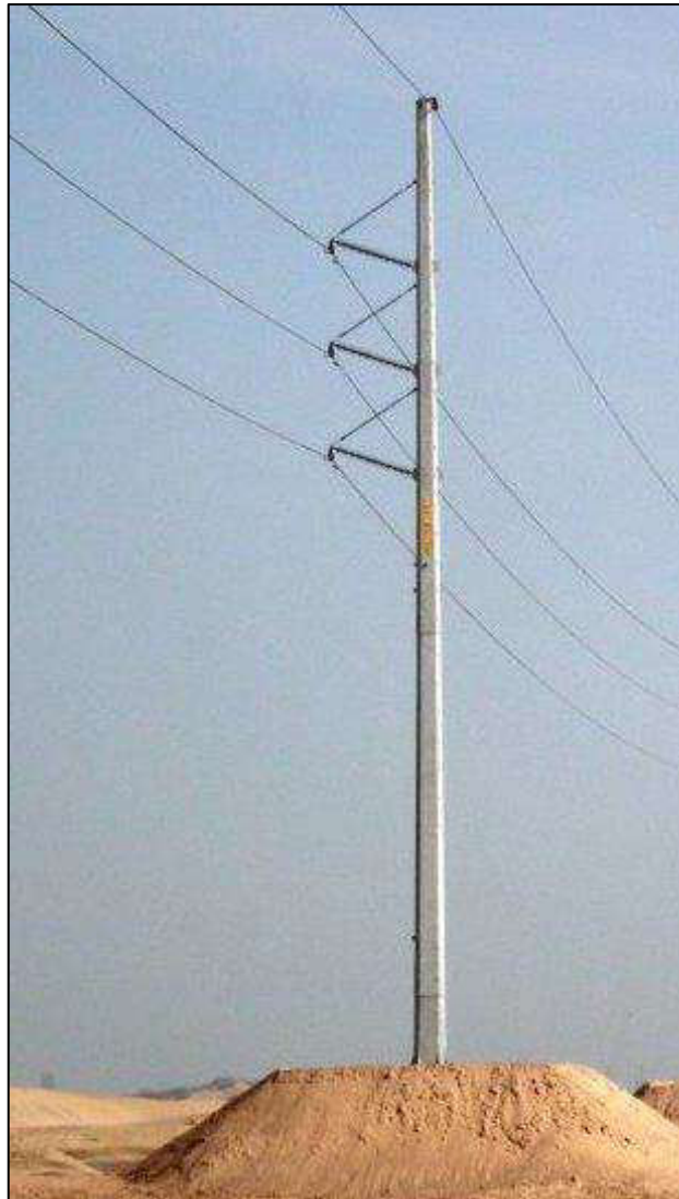
FIGURE 3: EXAMPLE OF A TYPICAL 132 KV STEEL MONO-POLE POWERLINE, SHOWING THREE CONDUCTORS AND AN EARTH WIRE ON TOP
