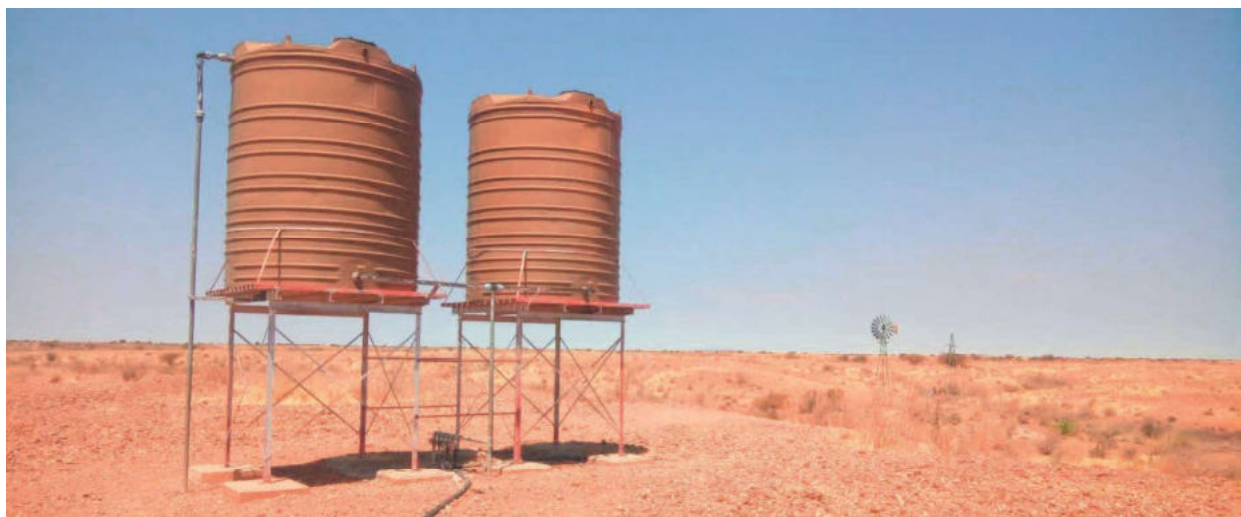
Figure 5: Shows the available water supply infrastructure (forefront, is the tanks and background Windmill)
