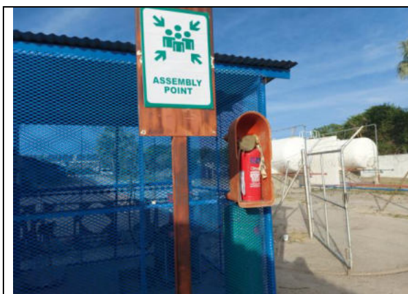
Photo 4-5 Fire extinguisher and emergency assembly point
