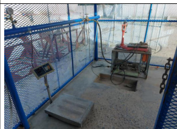
Photo 4-4 Cylinder filling area with scales
