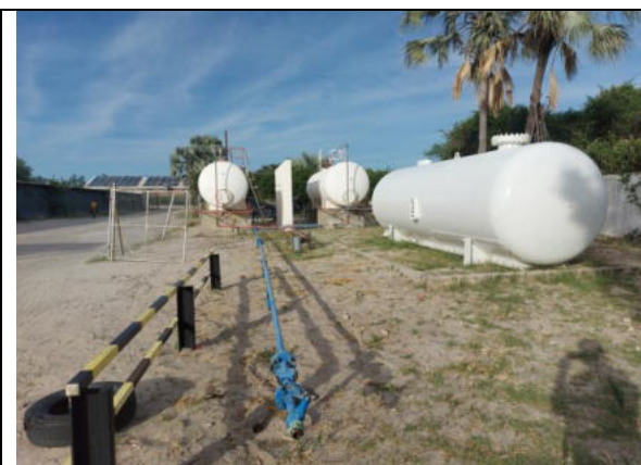
Photo 4-1 LPG storage tanks (back) and unused tank (front)
