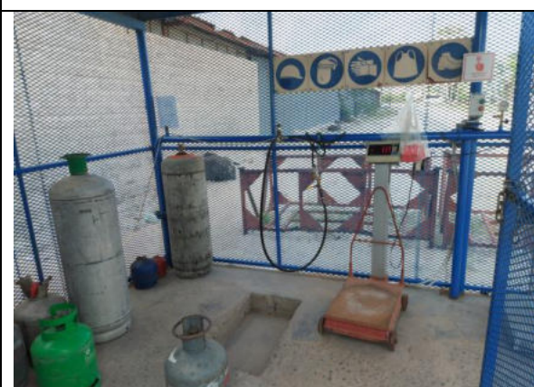
Photo 4-3 Cylinder filling area with emergency stop and PPE signage
