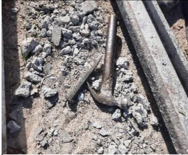
Defective tools observed onsite
