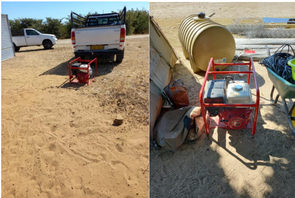
Figure 8 and 9 : Generators placed directly on the ground at Shiyambi and Masivi sites.
