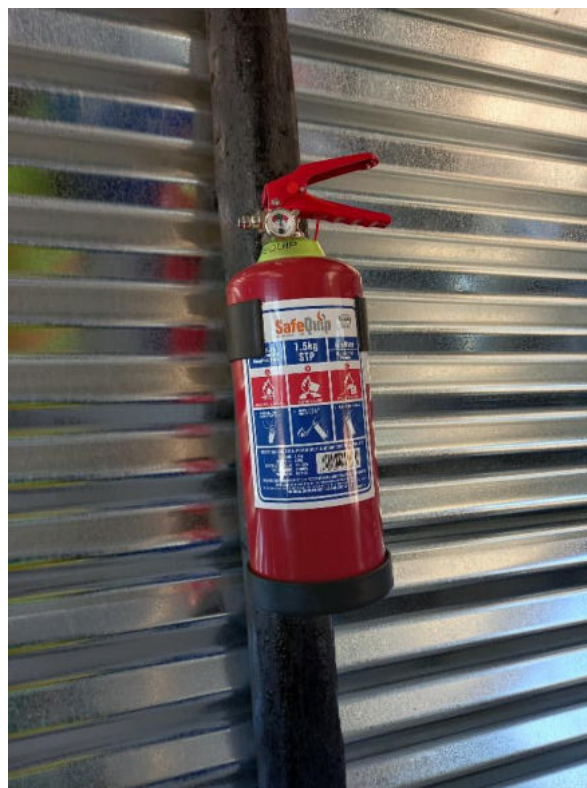
Figure 4: Fire extinguishers observed at both sites.
