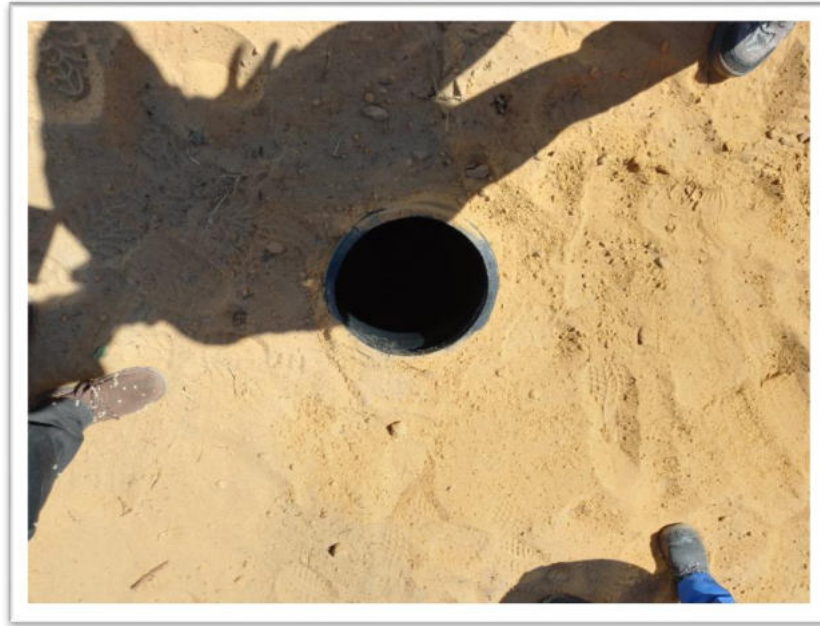
Figure 7 : Septic tank ( Demarcation or signage around the septic tanks to avoid to drive over incident) at both sites.
