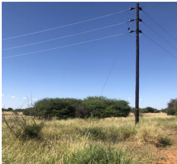
Picture 15 Electricity supply with CENORED infrastructure to site
