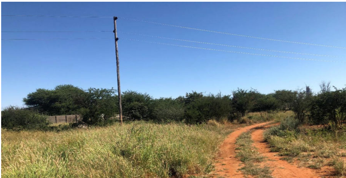
Picture 7 CENORED infrastructure/overhead powerlines adjacent to site
