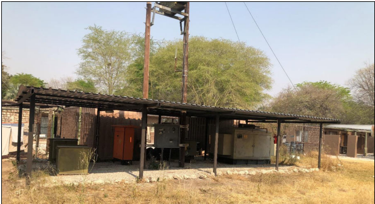
Figure 8: Electricity facilities on site
