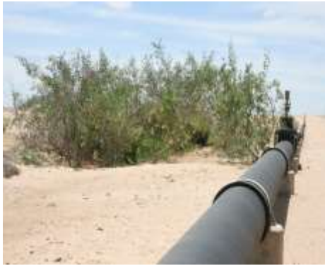
Figure 3: Nicotiana glauca associated with leakage along the aboveground section of the pipeline between the C14 gravel road and the Devils Fork junction 1 .
