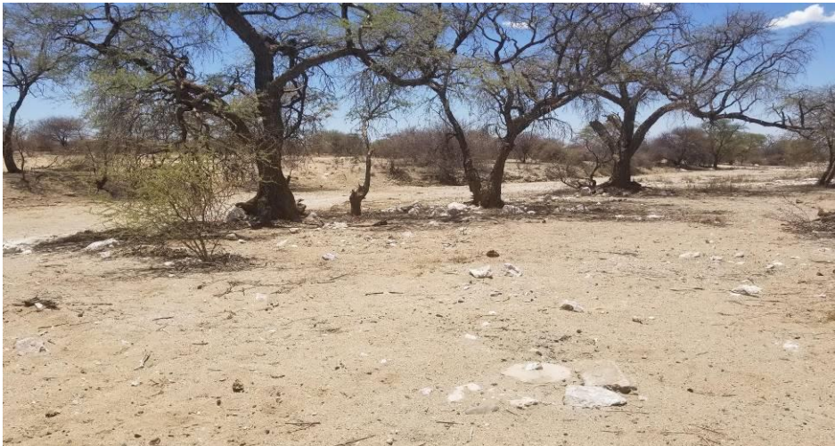
Figure 2 - Photo (DLE); prepared site (top), During drilling (middle), Cleaned up site after drilling (bottom)
