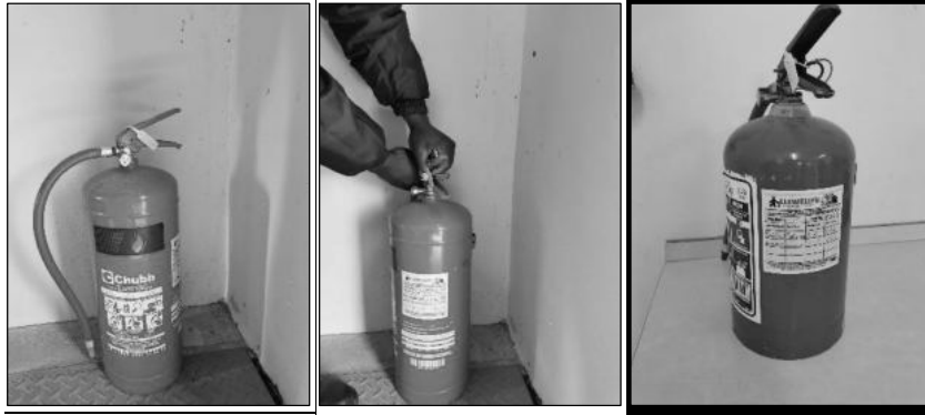
Figure 2-5: The fire extinguishers onsite
