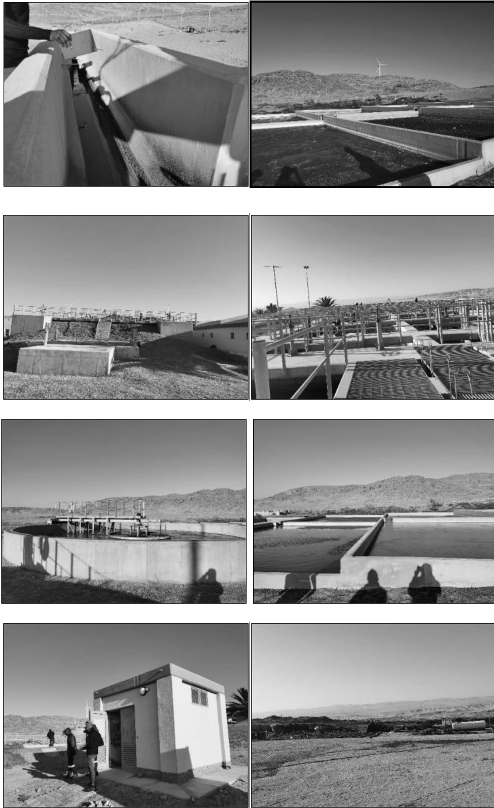
Figure 2-1: A view of the oxidation ponds, chlorine tank and associated infrastructure onsite
