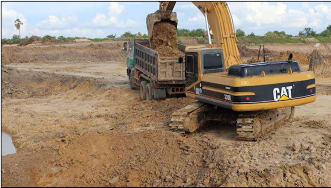
Figure 4: An excavator loading clay into a tipper truck in the quarry pit
