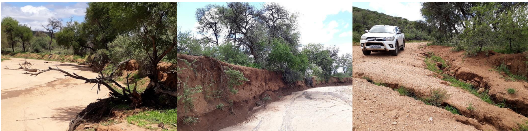
Figure 6: Pictures showing the eroded banks due to the recent flowing of the Usip River (the area had around 200 millimetres of rain since December 2019) (Source: L. Maartens, 25 February 2020).
