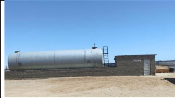
Photo 3-1 Diesel tank in bunding
