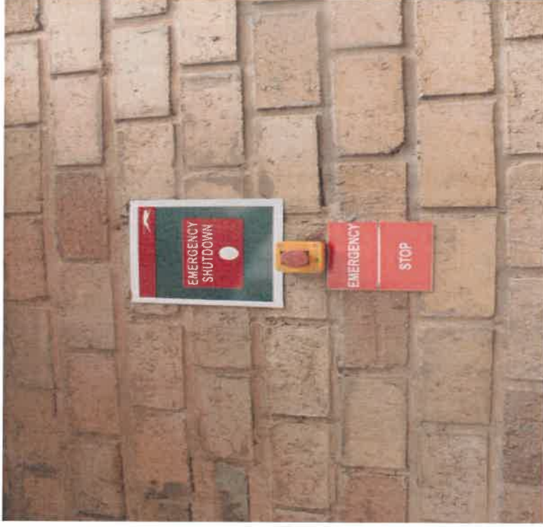
Figure 4; Emergency shutdown at the facility
