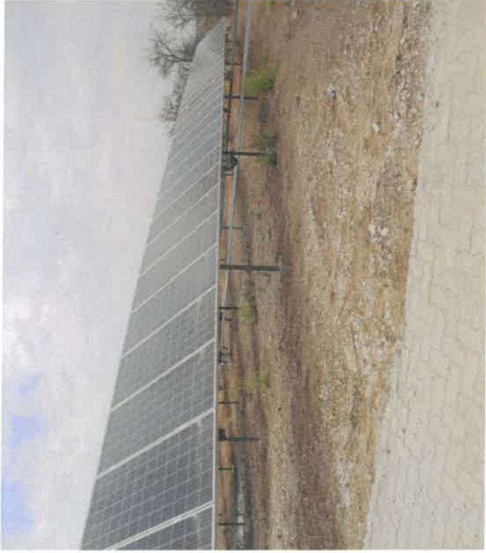
Figure 5; A solar power plant at the facility
