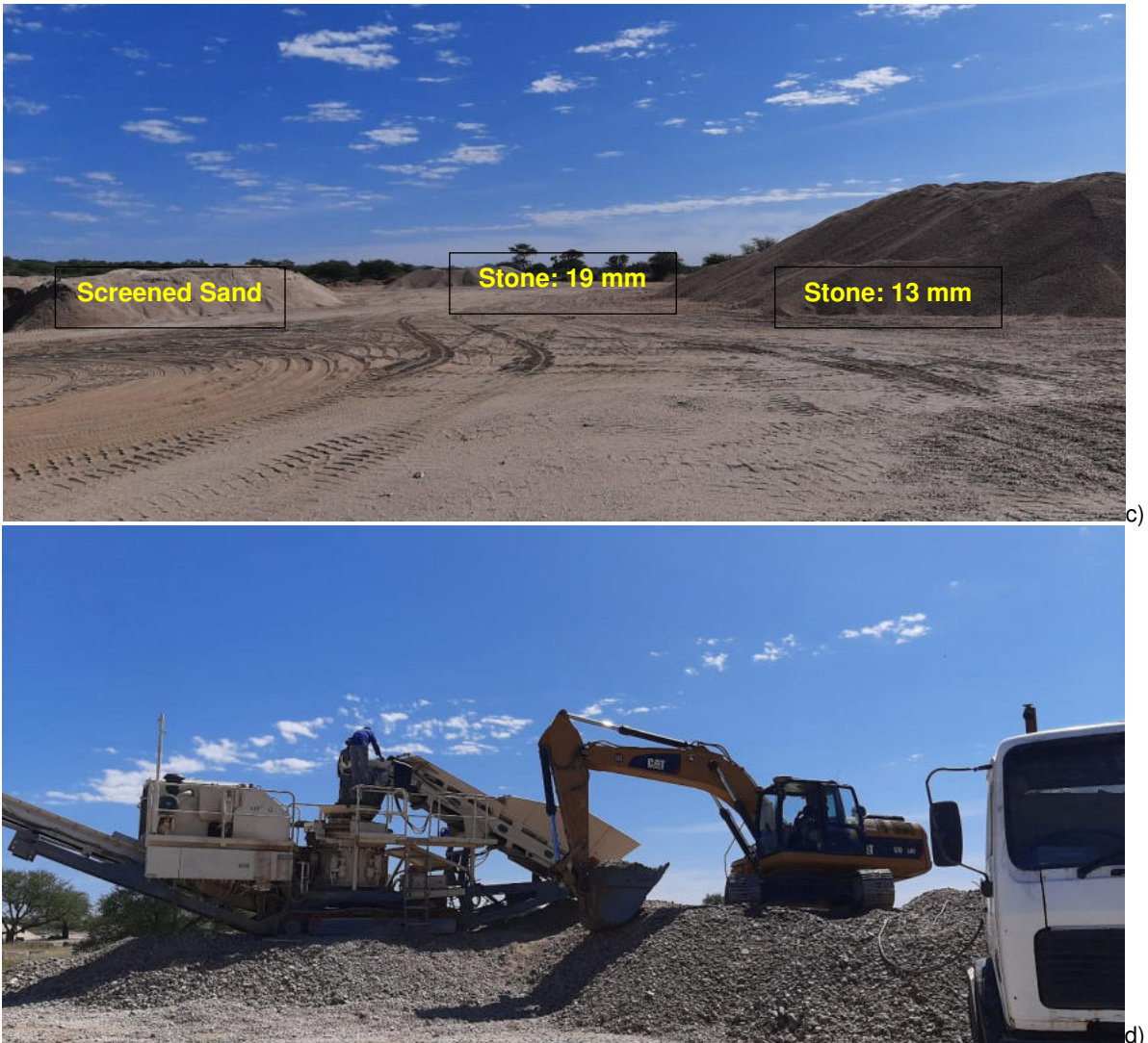
Figure 3: Pictures showing: a) junction of the river coming from Windhoek and flowing into the Swakop River; b) PowerScreen (the river sand can be seen in the background); c) the products: sand, 19 mm stone and 13 mm stone; d) an excavator in the process of loading oversize material onto the crusher ( Source: L. Maartens, 08 March 2023 ).
