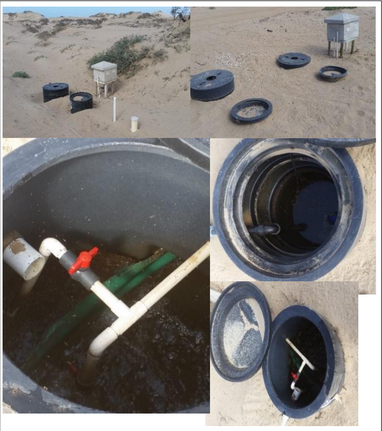
Figure 13. The Bubbler sewage treatment system: aboveground (top two pictures) and the insides of the breakdown and enzyme chambers (bottom three pictures).
