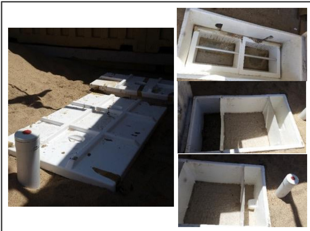
Figure 12. Fat traps at both the lodge kitchen and the staff kitchen.
