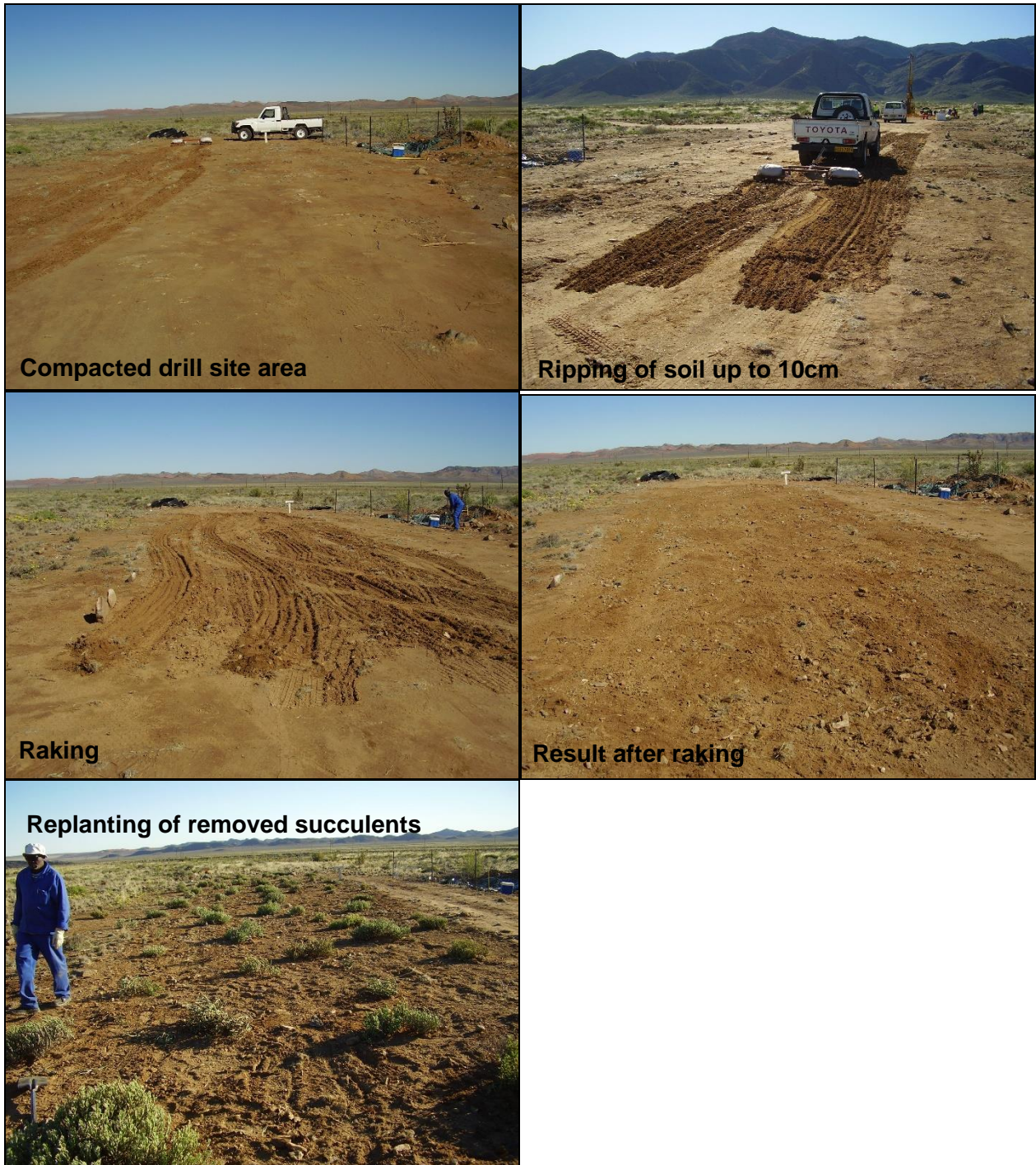
Plate 2: Example of rehabilitation of one of the access tracks created during drilling activities (January 2010).
