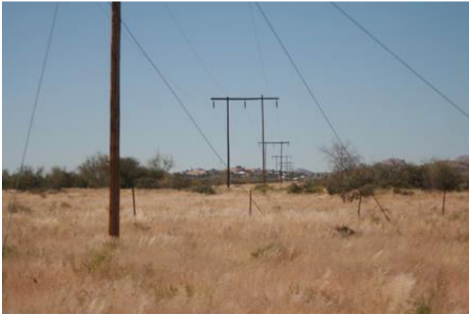
Figure 3. The 66KV Marble-Karibib transmission line with H-Pole structures.
