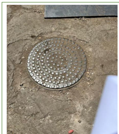
Photo 2. 23m 3 underground diesel tank
