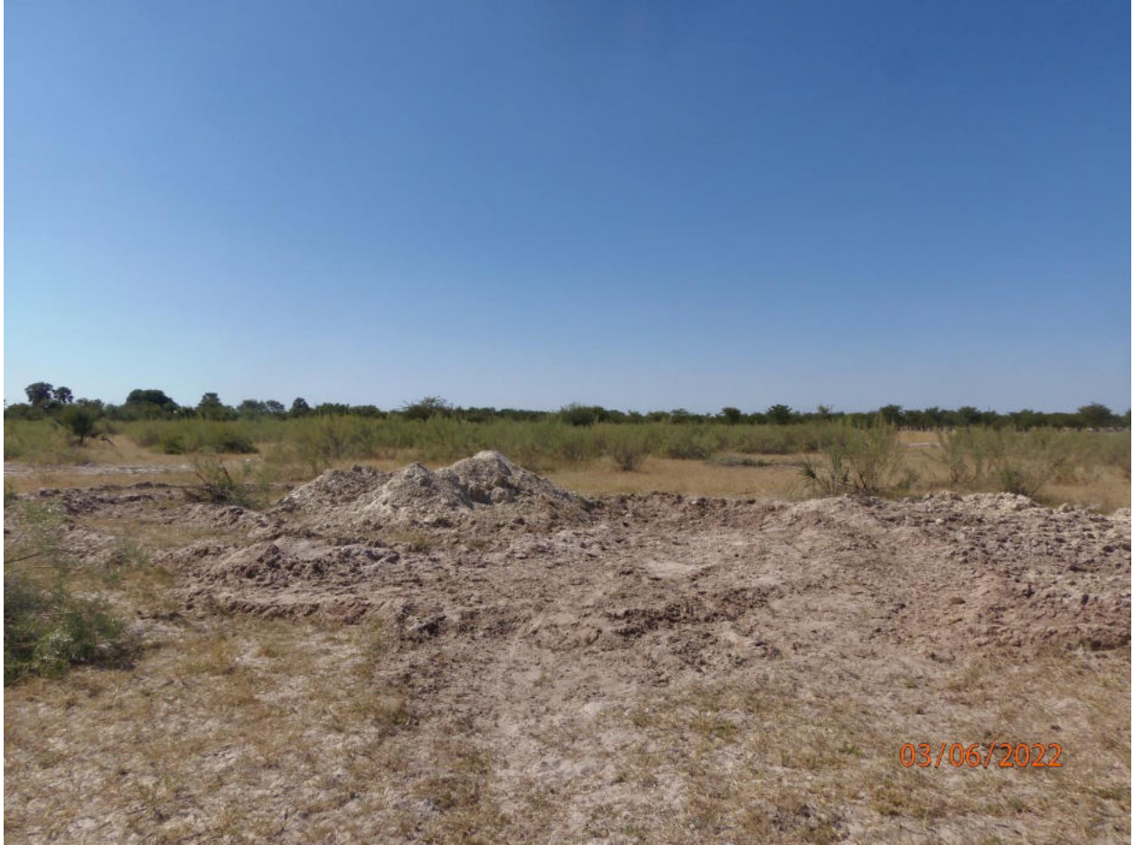
Trial pit for testing if the soil grade is suitable for road construction
