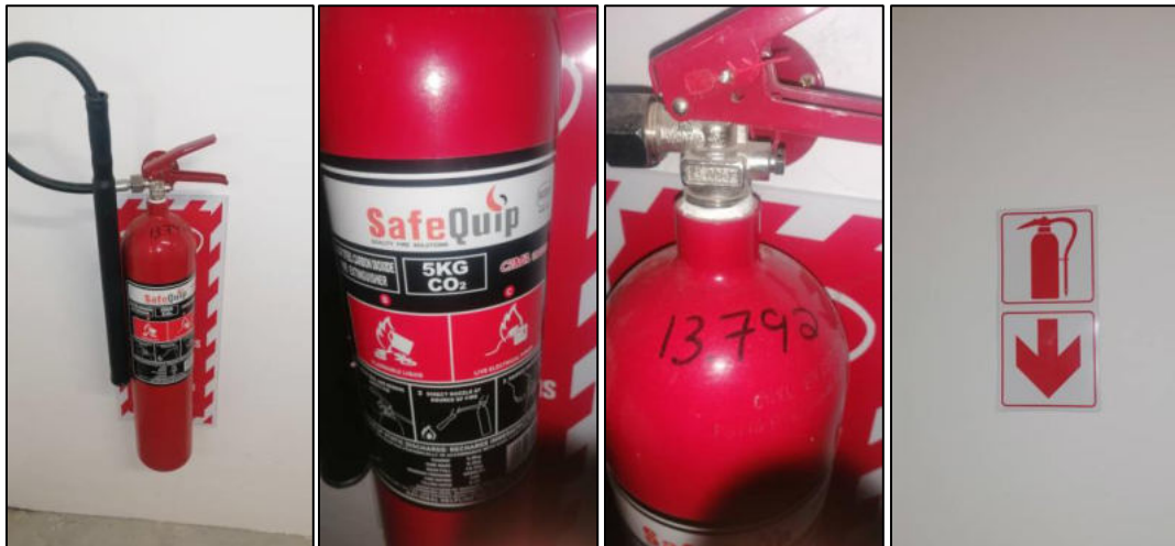
Figure 2-12: Fire extinguishing equipment in the site Office
