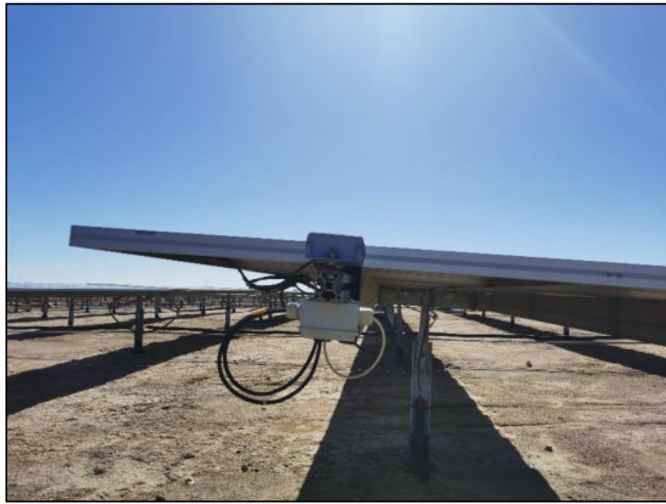
Figure 2-7: The sensor for detecting dirt on the panels
