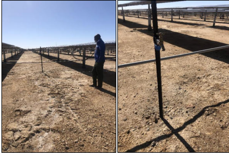
Figure 2-8: One of the Solar panels cleaning taps onsite
