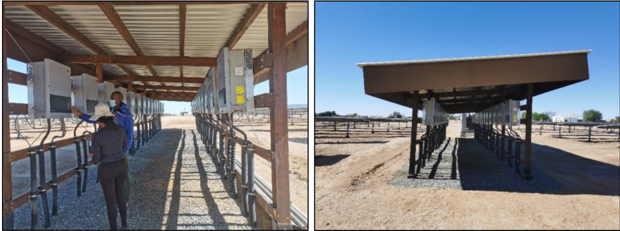
Figure 2-5: The Site inverters' substations (Substation 1 and 2) with the 30 inverters per Substation
