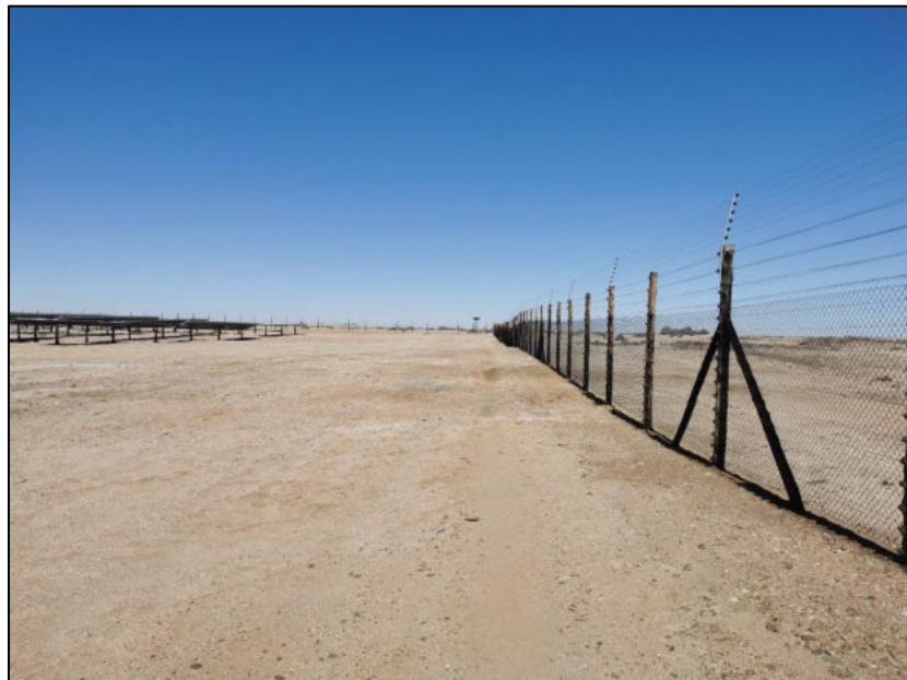
Figure 2-14: The 10m safety space between the western solar panels and the fence (view to the south). The inner fencing – electrical wire fence can also be seen on the right.
