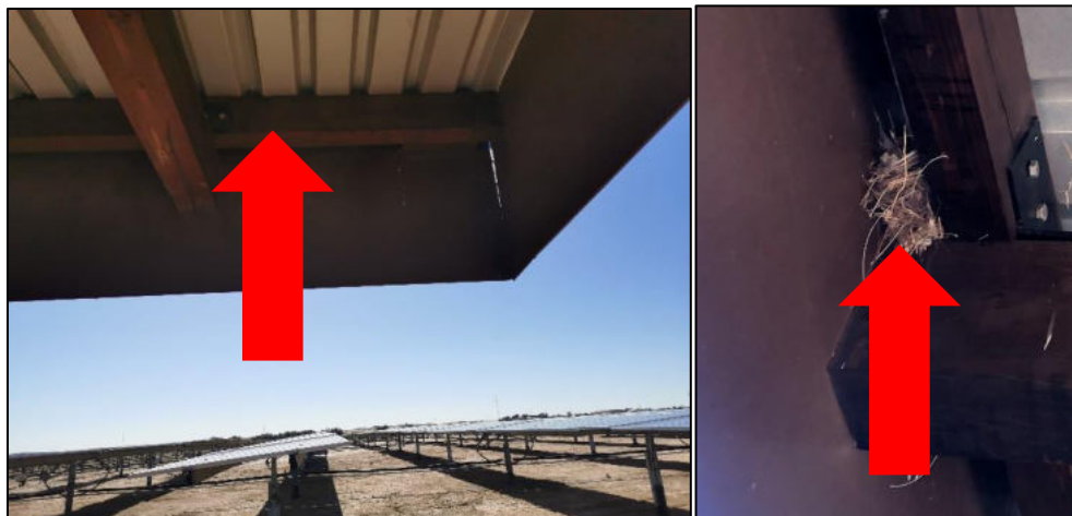
Figure 4-13: The Plant Substation roofs that houses the nests of some local bird species
