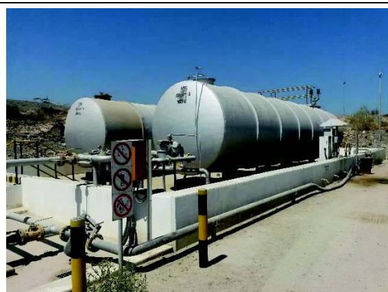
Photo 1 Existing diesel storage tanks
