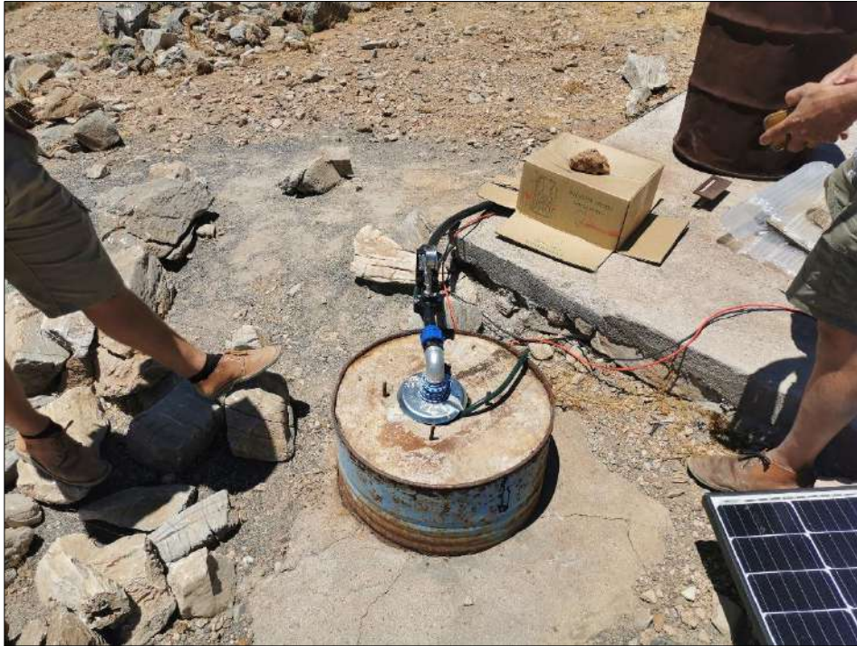
Figure 5-10: The solar powered borehole near the Camp site
